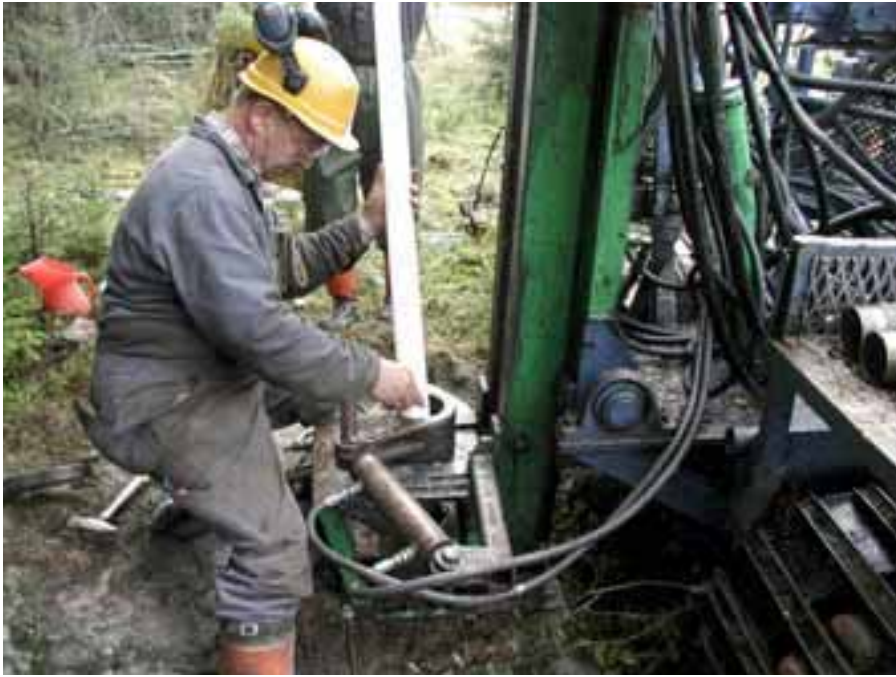
A total of 16 standpipes were installed in eight locations at Olkiluoto in autumn 2001 in order to examine the hydrological and chemical phenomena linked with the soil cover.
