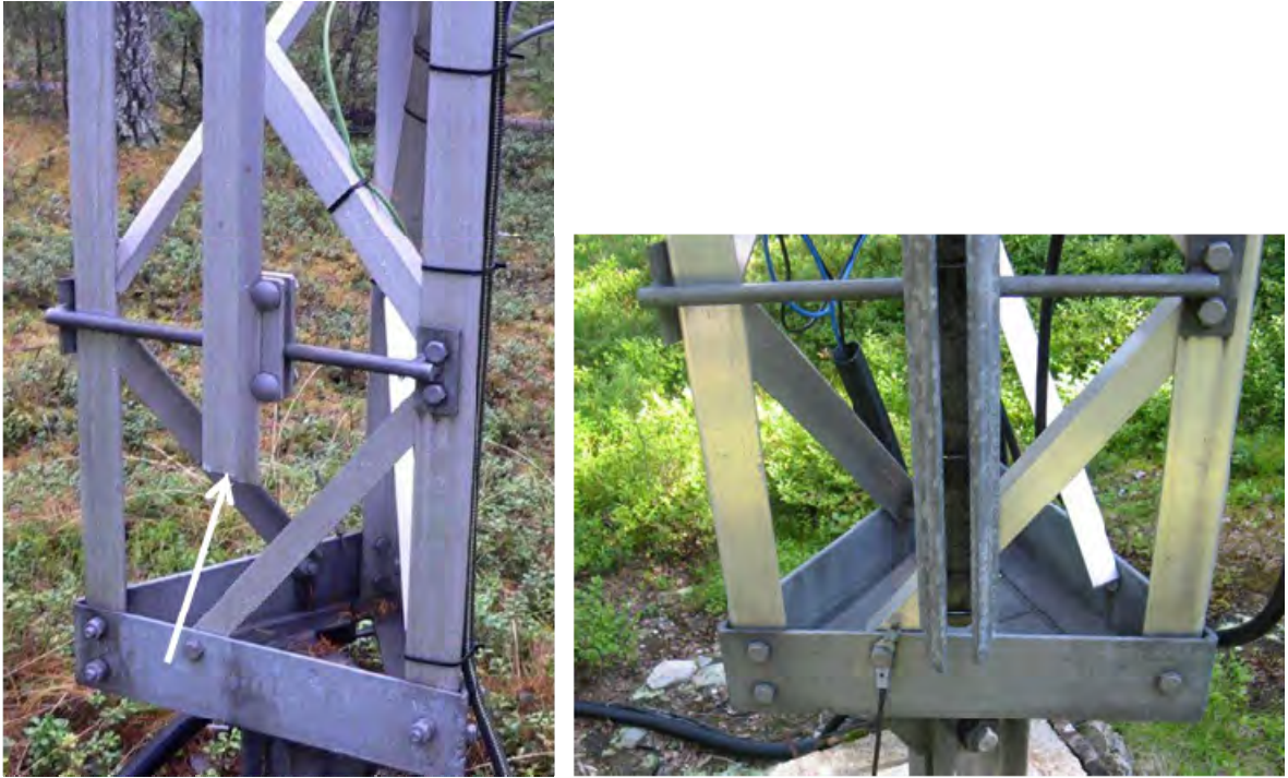
Figure 5. A vertical profile (left, marked with an arrow) was replaced with a newer model (right). Photos: A. Rynnänen/Luke.
