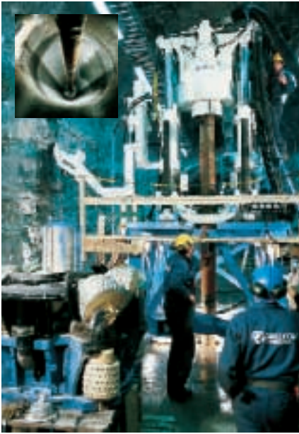
Deposition holes are bored into the floor of the final disposal tunnels respective to the fuel canisters.
