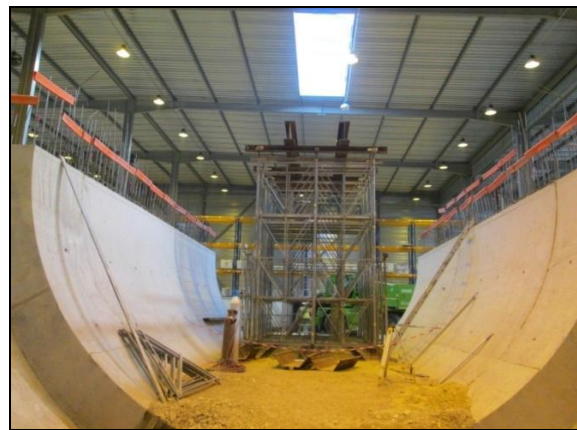
d) The completed lower part of the test box with a sand layer at the bottom and scaffolding also shown
