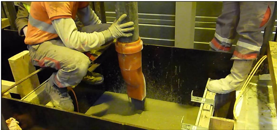
Figure 2.4: Test box used for metric-scale testing. In this photograph, the fluidity of the concrete is shown at the outlet of the pump and evidence of self-compaction is provided by the smooth surface produced (no vibration or shocks were applied during the test) (Bosgiraud and Foin, 2014).
