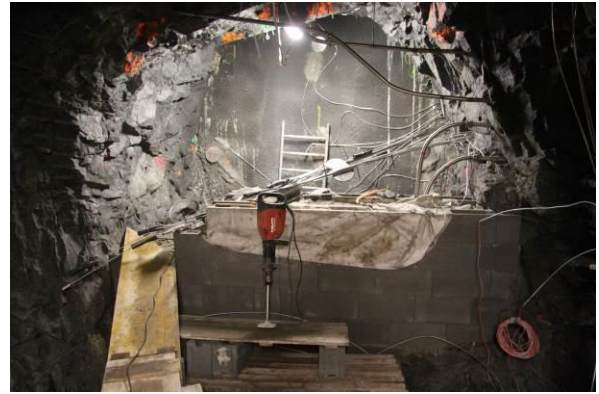
First part of filter erected (photo taken at the start of bentonite installation, 5.6.2015)
