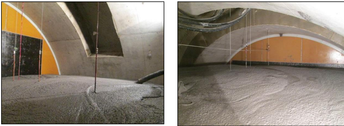
Figure 2.11: Pouring and even emplacement of SCC inside the test box (left) and emplacement of SCC close to the recess (right) (Bosgiraud and Foin, 2014).
