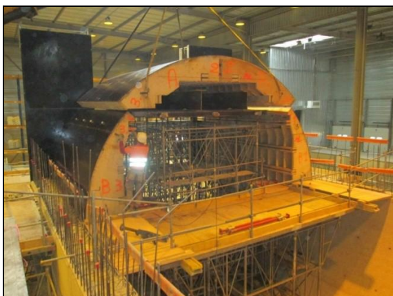
e) Removal and translation of the wooden formwork between the two phases of the upper block casting
