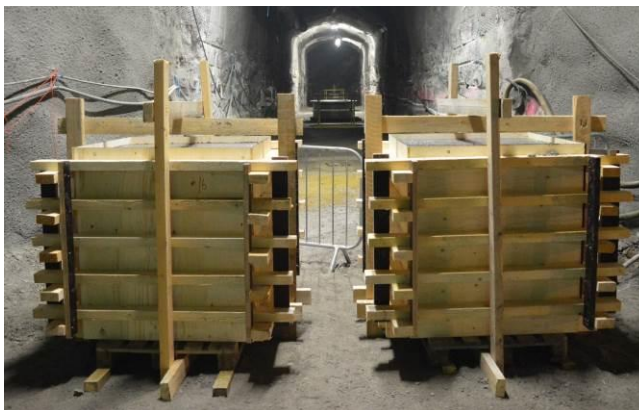
Quality control 1 m 3 cubes for 16 and 32 mm aggregate mixtures, Concrete Wedge Section One.
